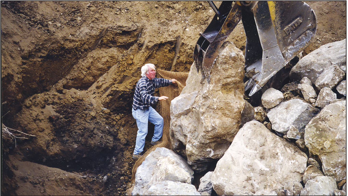
Randy Young vs. Pac-Man as the long hydraulic arm of an excavator moves boulders into place in the Los Lions catch basin just north of Sunset Boulevard in 1998.
