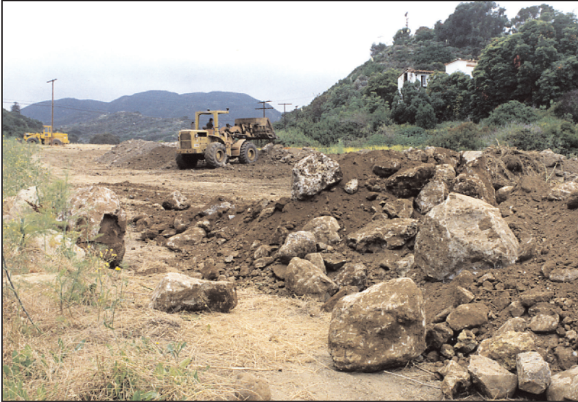
In 1998, two thousand tons of Chico conglomerate from the La Tuna Canyon slide and cut (valued at $100,000) were donated by Caltrans and delivered to lower Los Lionses by L&T Excavating. The rock was used for lining the half-mile stream channel, stabilizing canyon slopes, and decorating the facilities and walls. Photo: Pacific Palisades Historical Society
